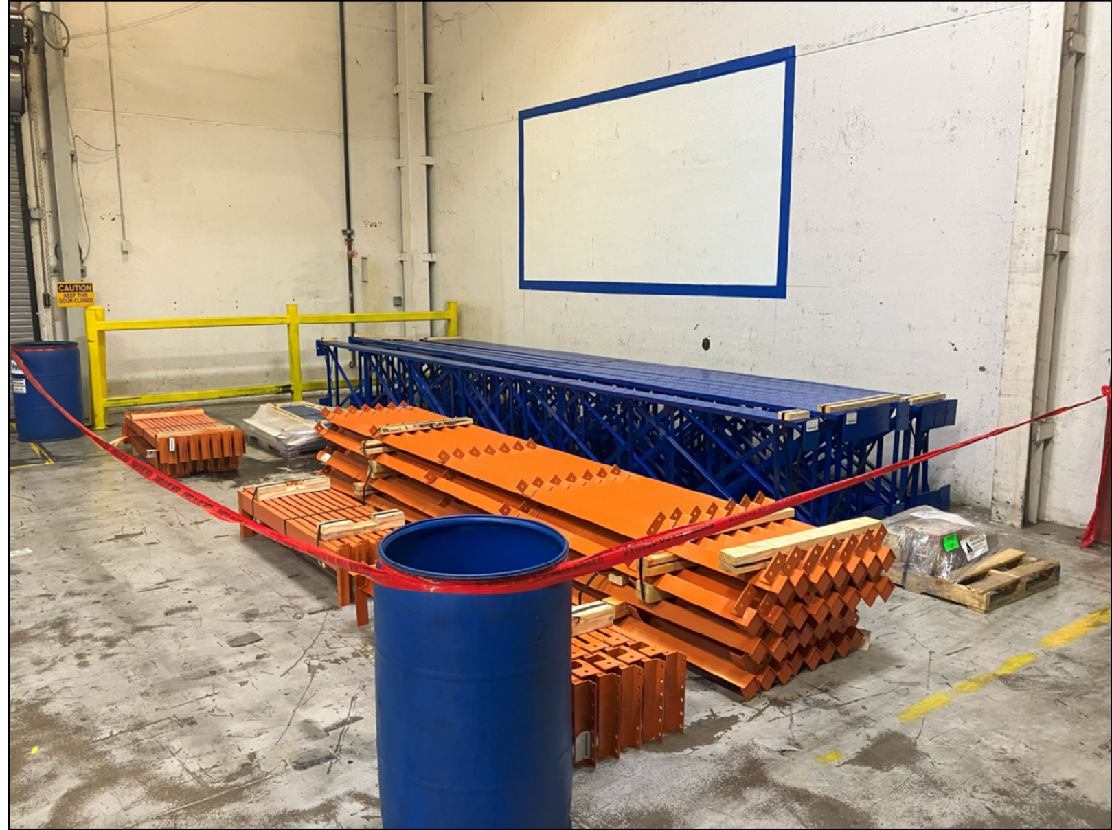
Staged the drive-in rack system in the area that it's going – CORDONED OFF – KEEP OUT!
