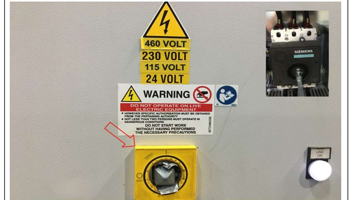
REPLACE BROKEN DISCONNECT HANDLE ON MAIN PANEL BOARD
