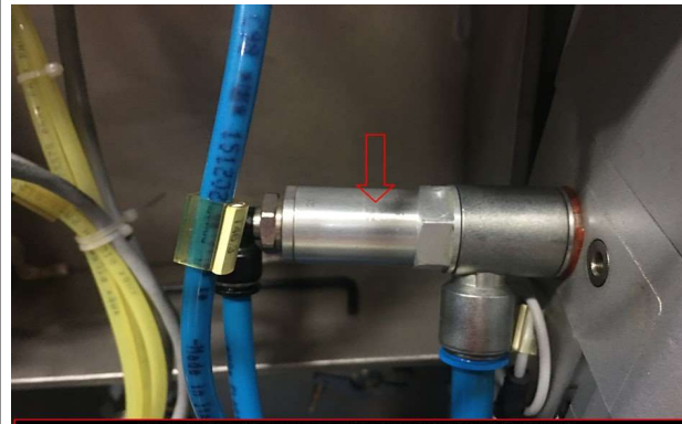
REPLACE BOTH DEFECTIVE DOOR CONTROL VALVES
